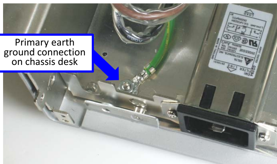
Figure 90 Measure the resistance from the power supply enclosure to the primary earth ground connection on the chassis deck.
